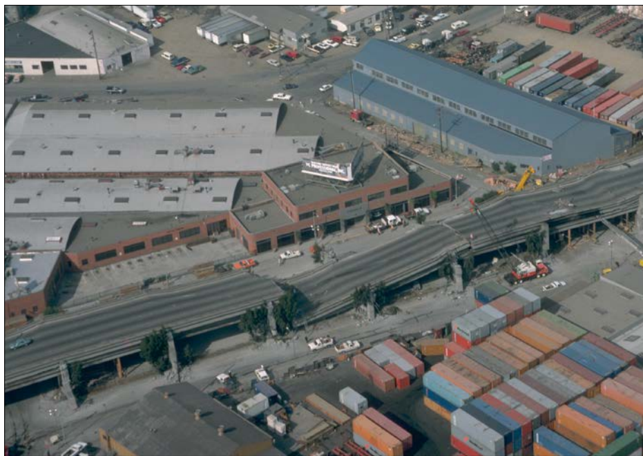
The upper deck of the Cypress Street Viaduct sheared off of its support columns and collapsed onto the lower deck. The soft soil around the viaduct's foundation amplified shaking, contributing to its collapse.
