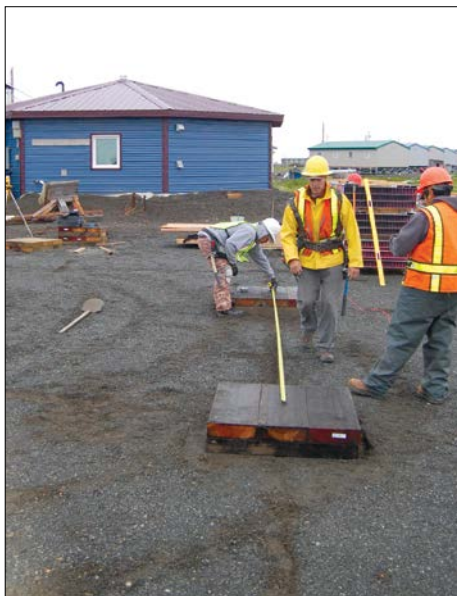
Efforts to enhance energy efficiency, as in the Quinhagak prototype designed by the Cold Climate Housing Research Center in partnership with the Native Village of Kwinhagak, reduce a household's utility costs, which in turn can make homeownership more sustainable.
