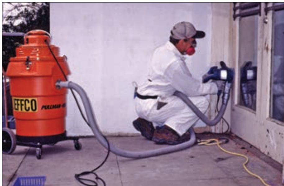
Appropriate precautions must be taken when working with lead-based paint. Here a worker uses a sander attached to a high-efficiency particulate air-filtered vacuum.
