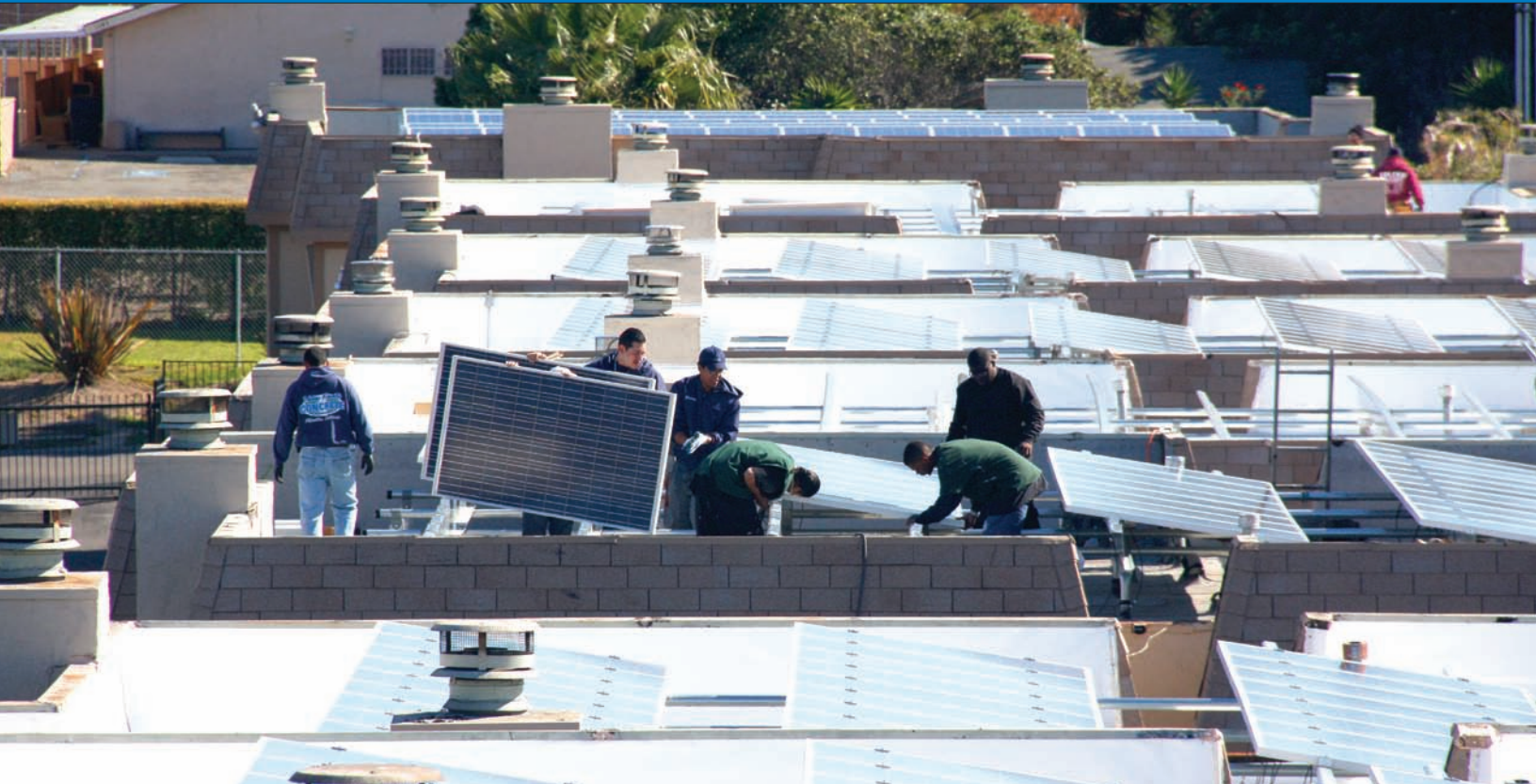
Young adults from the YouthBuild program equip multifamily housing buildings with solar panels while learning to install the new technology.
